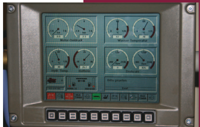
Board Control System
