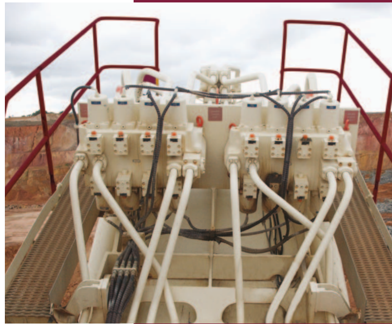
Main hydraulic valve block
